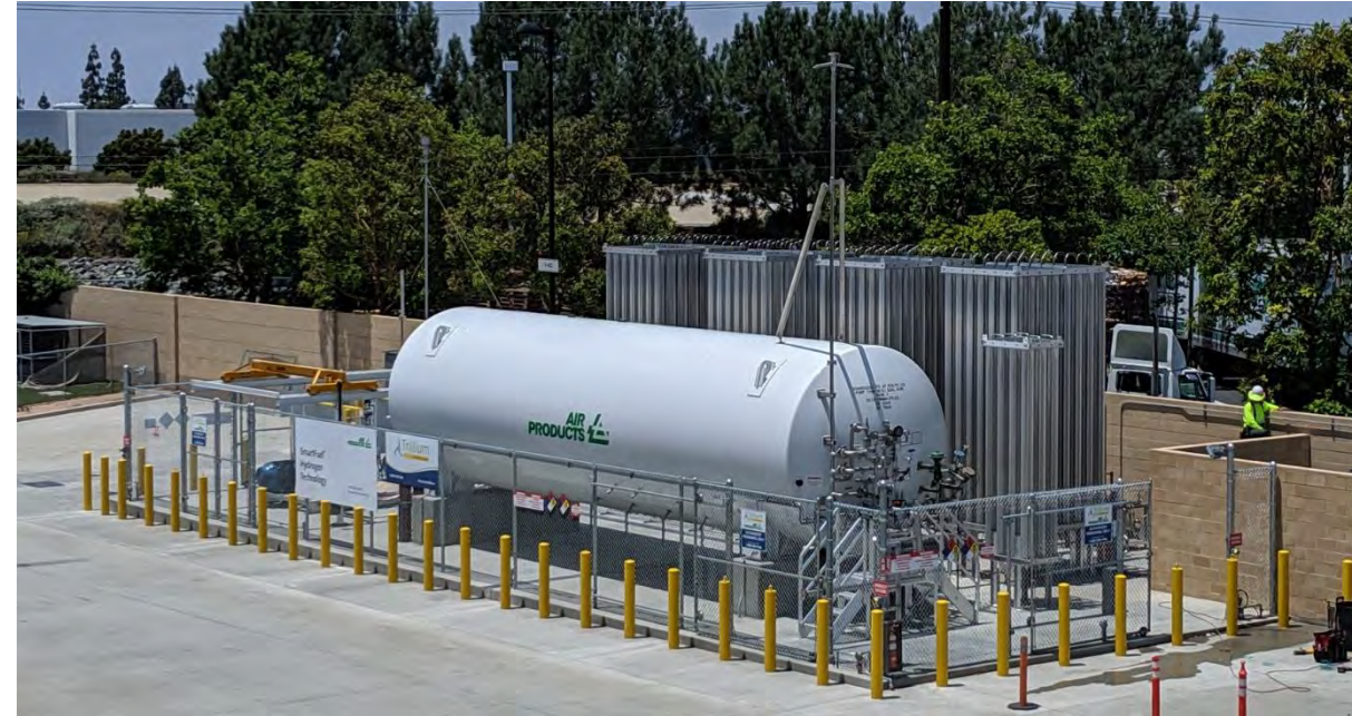
Hydrogen Fueling Station
