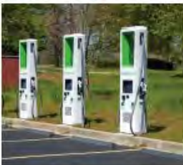
Electric vehicle charging
