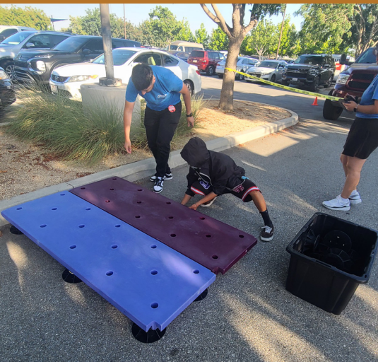
The project team, with assistance of some volunteers, built a temporary curb extension.
