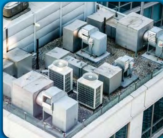
Commercial Combustion Water/Space/Heating/ Cooking/Others
