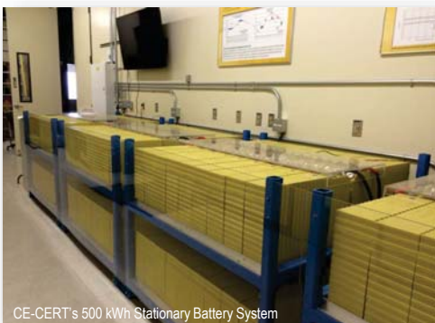
CE-CERT's 500 kWh Stationary Battery System
