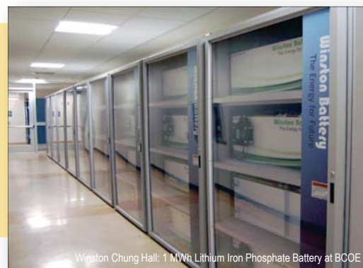
Winston Chung Hall: 1 MWh Lithium Iron Phosphate Battery at BCOE
