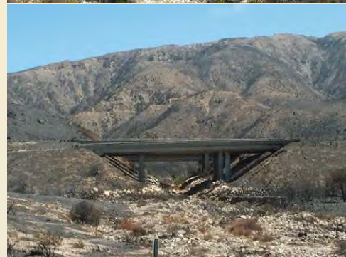
Bridges on I-15 north of Cleghorn Canyon; the top is 0.7 miles north of Cleghorn; the bottom is 400 yards south of the Cajon interchange.
