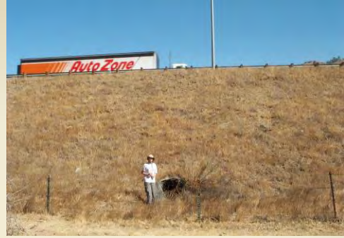
Fill slope along SR-58 that should be replaced with a bridge.
