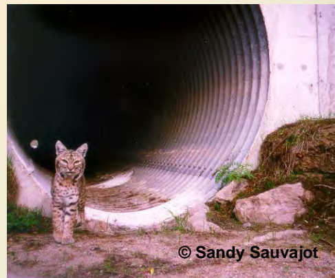
Pipe culvert north of Tierra Rejada; typical of most structures on SR-23.
