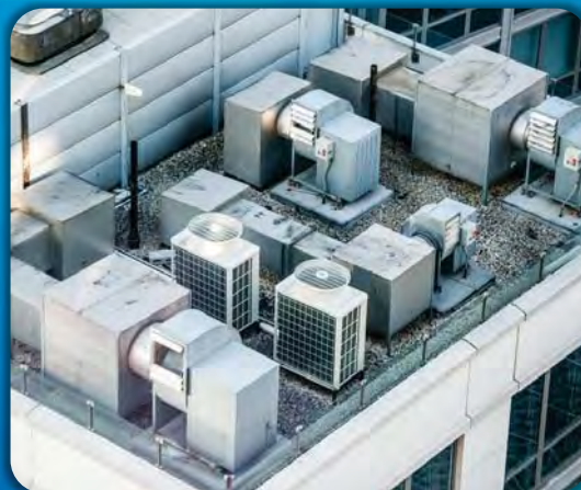
Commercial Combustion Water/Space/Heating/ Cooking/Others
